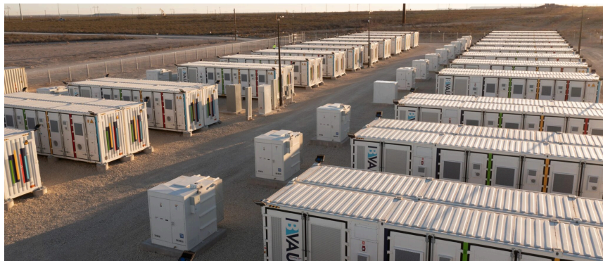
Battery energy storage by Energy Vault Energy Vault
